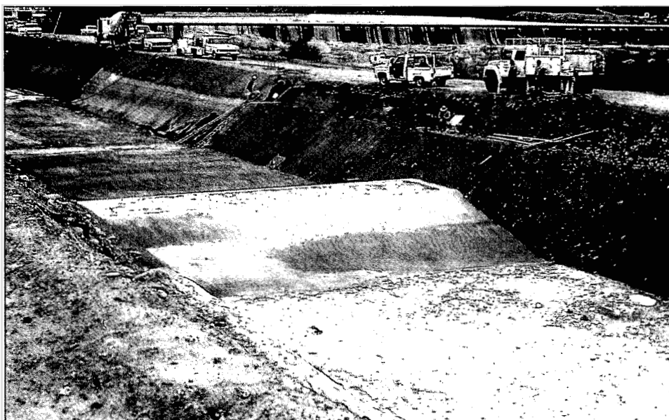
Figure 1.9 This 15.45 m wide flume has a throat length of 3.05 m. At its design capacity of 56.6 m 3 /s, a head loss of only 0.12 m is required for flow to be modular. On large structures, a 6:1 downstream ramp truncated at half the total drop height reduces construction cost. Low crests (<0.5 m) often have a vertical downstream face (Arizona).
