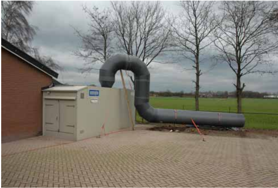
Figure 5.4 Funnel on top of the droplet remover from a combined air scrubber to slow down the air speed
