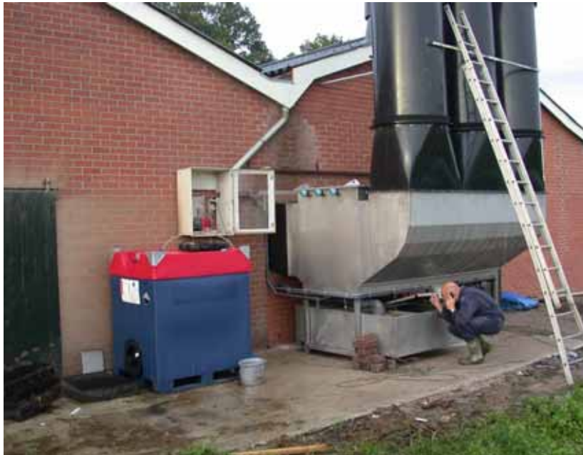
Figure 5.1 Chemical air scrubber next to an animal house with circular ducts for the outgoing air
