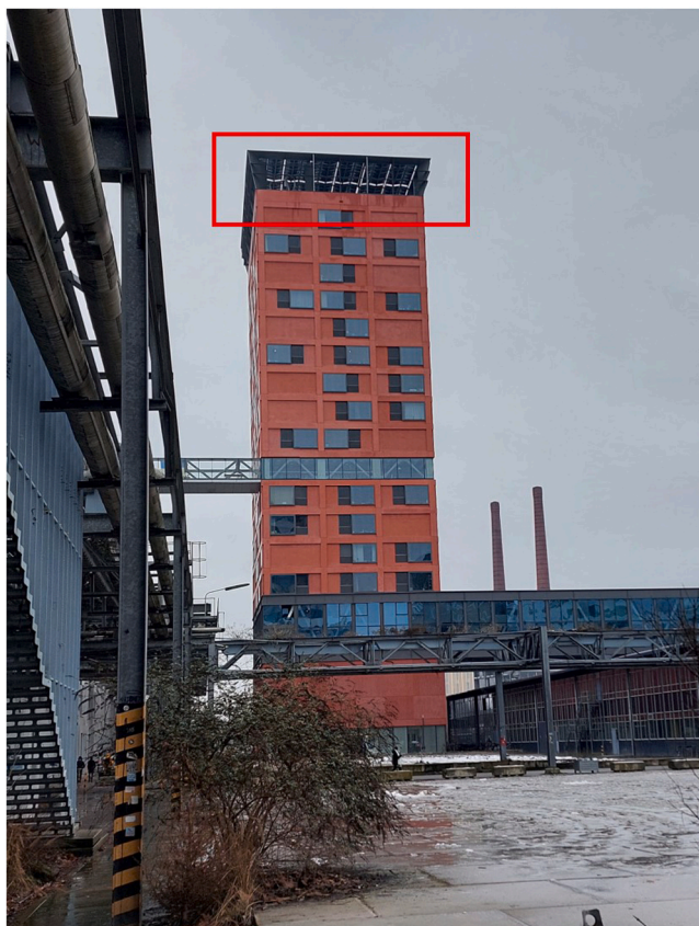
Fig. 3. Power Nest system on a building in Eindhoven, the Netherlands (the picture was taken by the first author).
