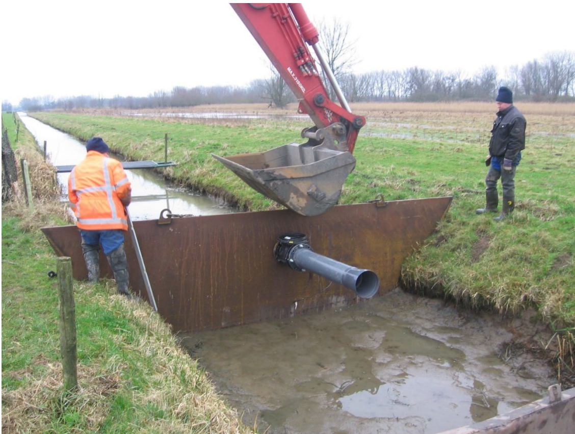
Figure 11 Weir E including electromagnetic flow meter placed into the ditch.
