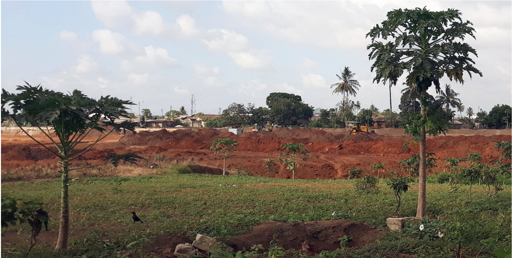
Photo 4. Agricultural plots are left fallow after the last harvest, while in the background a bulldozer is levelling the agricultural fields for construction (23-11-2021).
