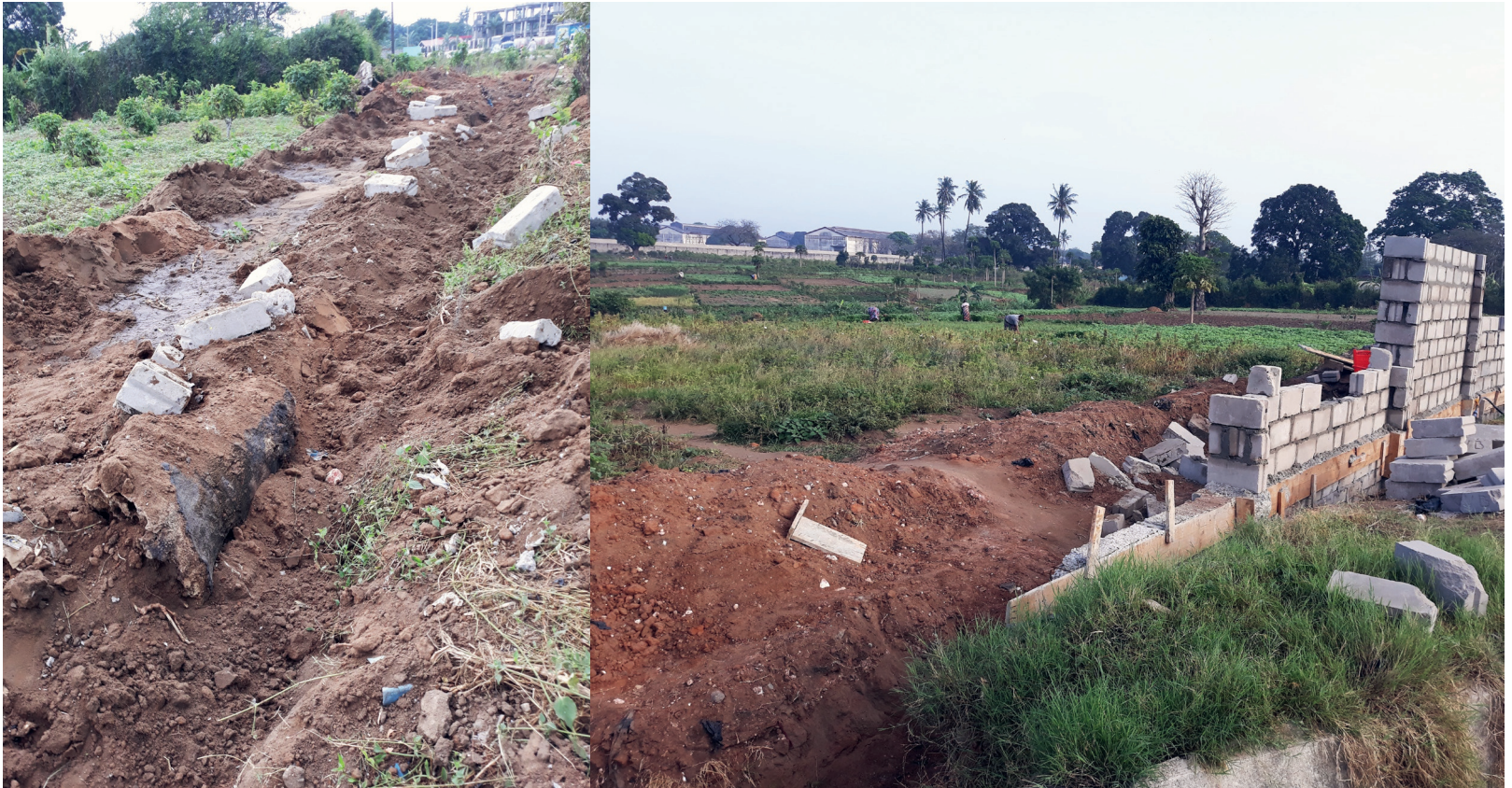
Photo 2. Excavated trench that is backfilled and building blocks that are demolished out of protest against the planned development of the area (15-07-2021). Photo 3. Wall construction is underway while farmers in the background harvest their last crops (17-08-2021).
