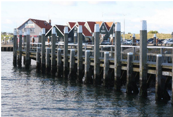
Figure 6 Mooring-posts in the harbour of Oude Schilt, Texel. (Photo Eric de Munck, CentrumHout)
