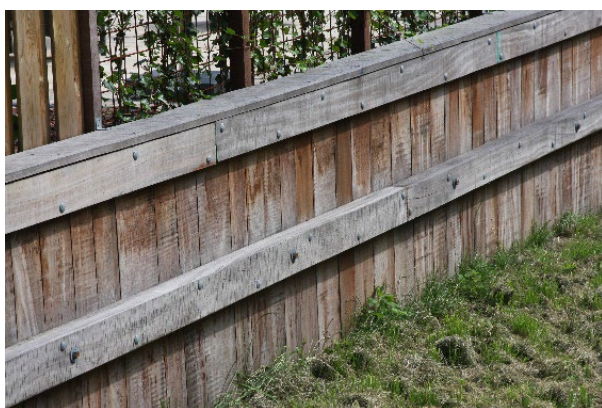
Figure 4 Double girdle mounted on sheet pile planks. (Photo Eric de Munck, CentrumHout)
