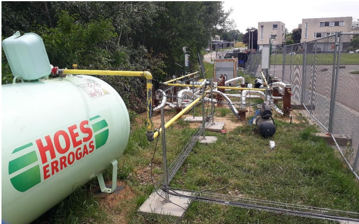
Figure 5. In situ installation of HAEMERS Technologies in Heerlen. Eight smart burners were installed to treat the soil of a site infested with Japanese knotweed
