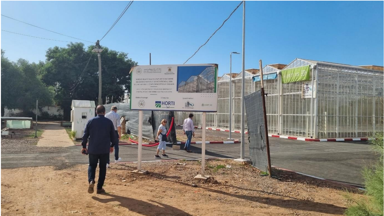
Current status of the greenhouse: almost finished but just not. Irrigation lines and substrate are not yet there, the head grower has been appointed on Dec, 1 st , 2023.
