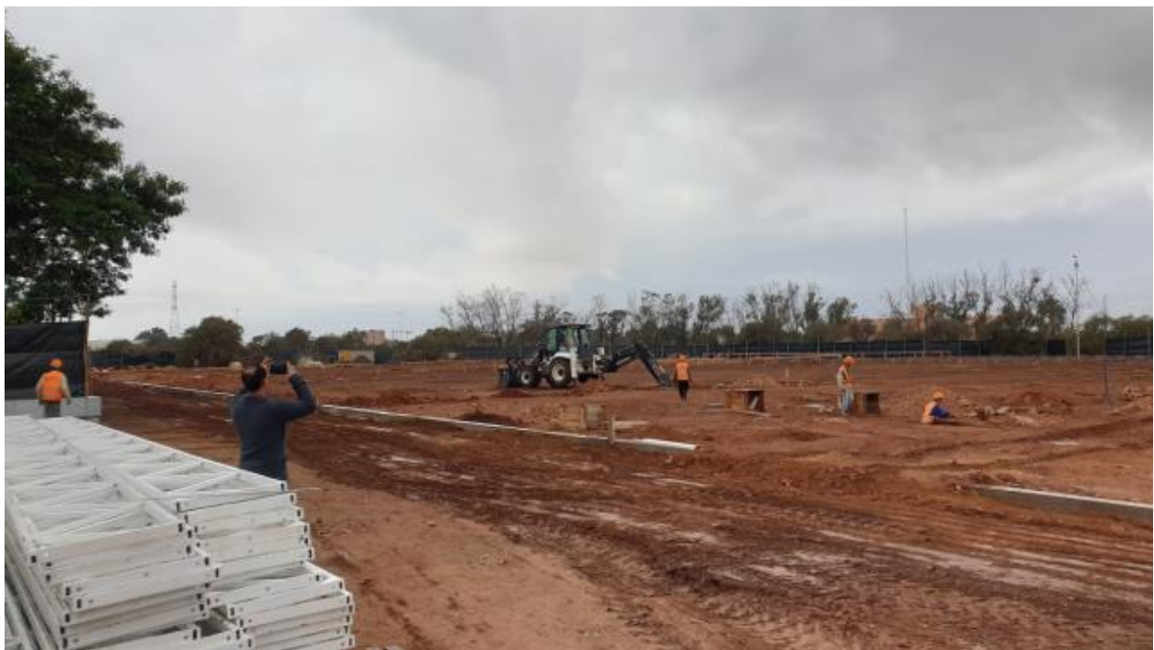
The picture shows the current (14-03-2022) of the construction of the center. The steel construction is present and well as the glass for the covering of the greenhouse.
