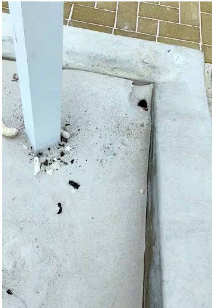
Figure 5. Sand can be seen accumulating along the retention wall.
