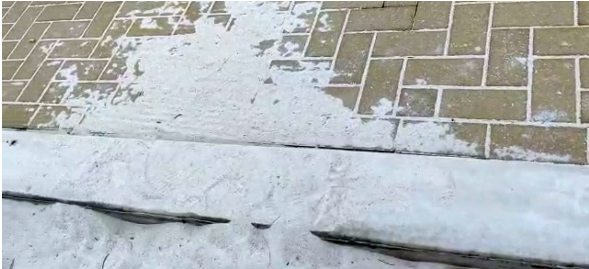
Figure 7. The sand in several places is already being transported over the edge of the wall.
