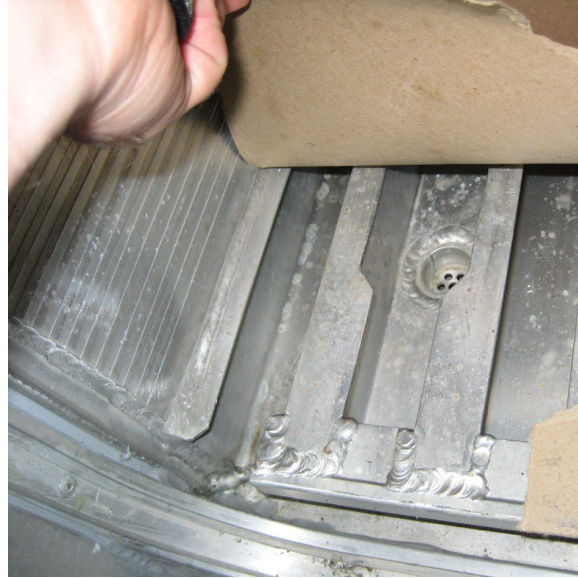
Drain hole needs to be closed!
