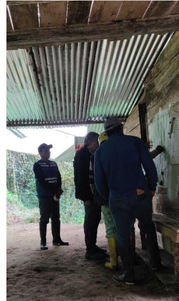
Image 8: Planning the day at the project site with Craig, his employees and the ground manager.
