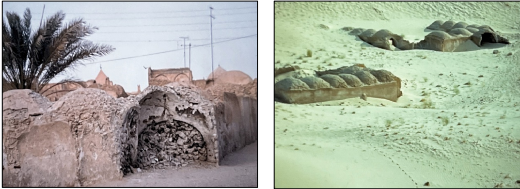
Figure 8. Deterioration (left) and burial (right) of traditional housing in the town of Gumar, Algeria (photos: M. Sherzad).
