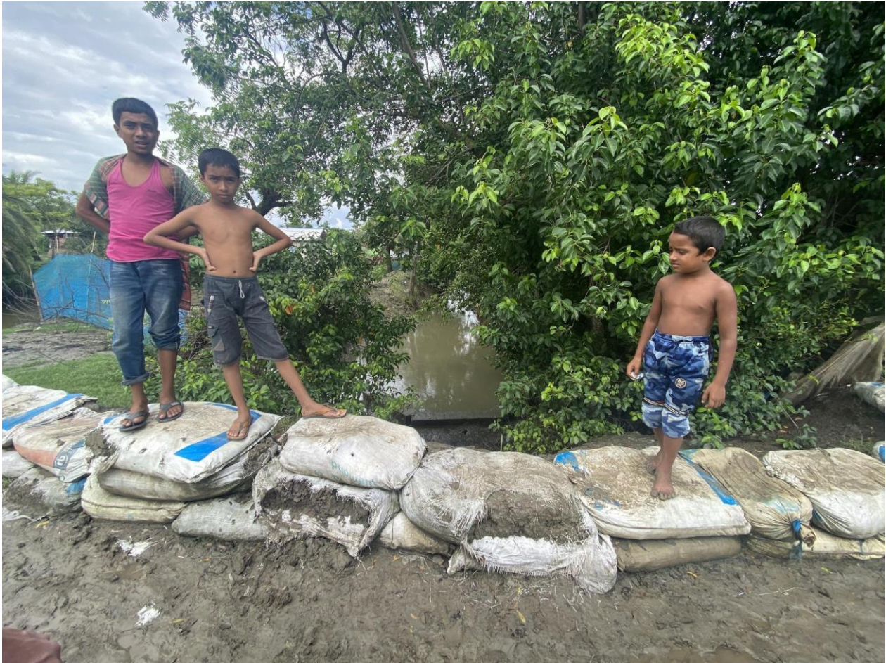
Figure 22 The outlet of the concrete pipe is shown in the picture, also the sandbags that are used to increase the height of the embankment and protect it from an overflow of water. At the other side of the embankment, not visible in this picture, the canal in the micro-watershed starts.
