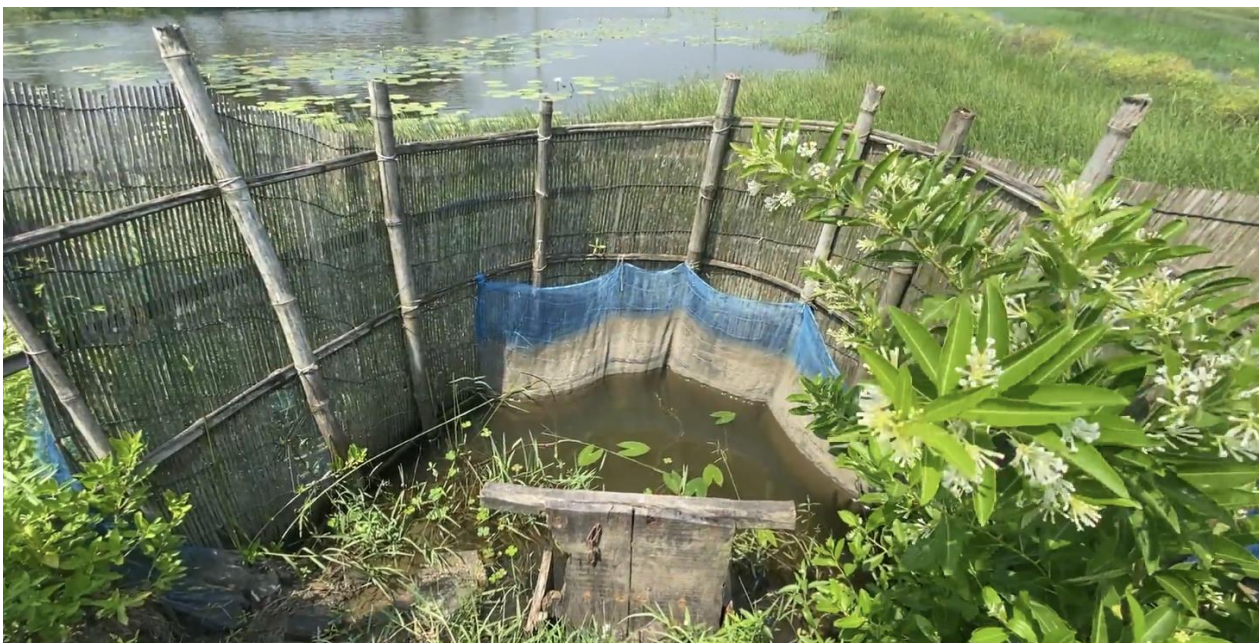
Figure 11 Wooden sluice gate to control water flow and bamboo fence to restrict the movement of fish outside canal.
