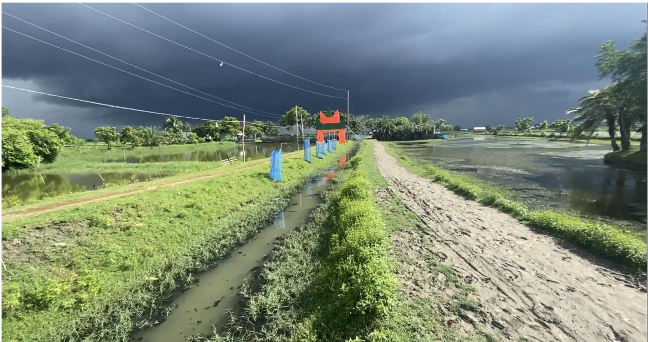
Figure 19 Severe siltation in the canal that was re-excavated in Pilot 3.
