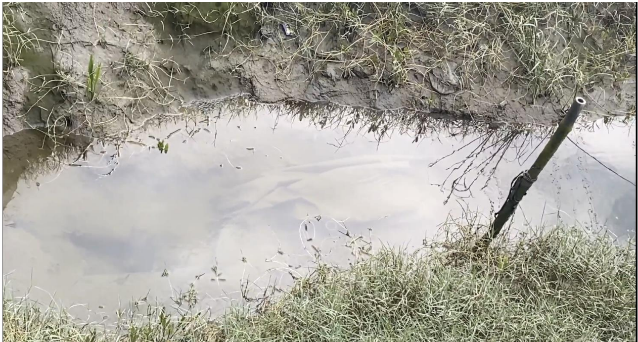
Figure 18 Pipe installed on the inlet pipe of the re-excavated canal. This structure allows drainage of water, but restricts entry of water into the micro-watershed.
