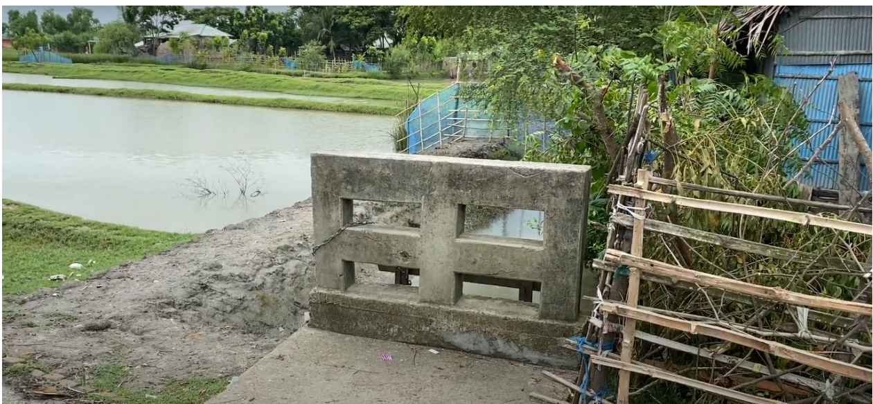
Figure 32 Sluice gate for controlling water flow in and out of the micro-watershed.
