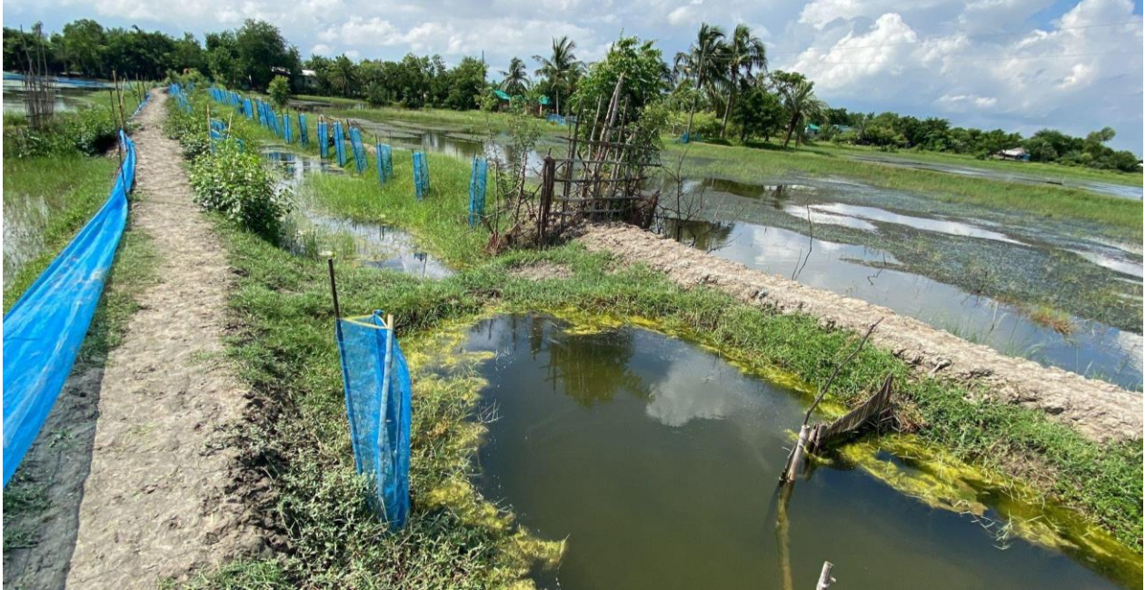
Figure 25 Re-excavated canal in Kalabaria in pilot 3, Debhata, Satkhira, Bangladesh. Additional information on the picture: Part of the restored canal, mangroves, and ponds can be seen in the image. A temporary bridge for transportation has been made, which has a pipe for water flow. The structure to capture fish, in the bottom right, has been folded based on the decision of the local water management committee to fold it to increase the water-carrying capacity of the canal.
