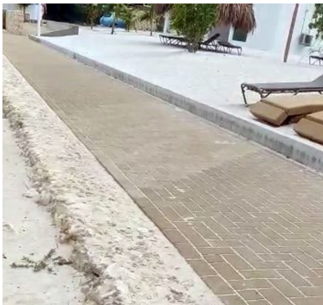
Figure 3. Footpath with retaining wall on the right side. Artificial beach sand is on the right side of the wall. Some natural sand is visible on the left of the picture.
