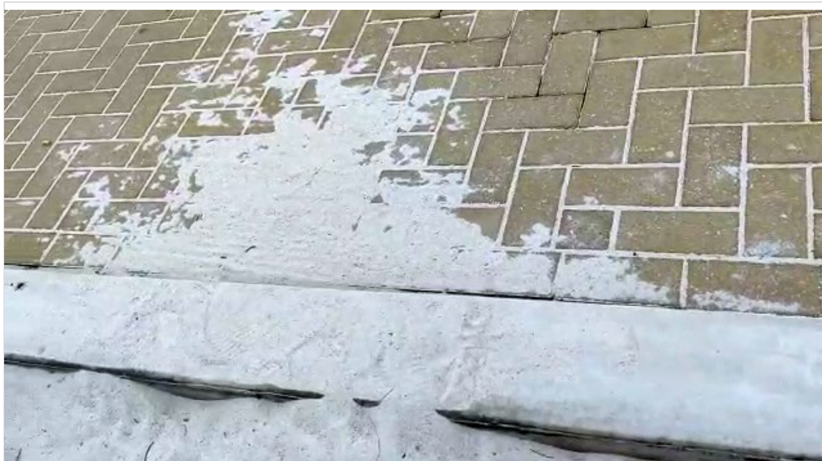
Figure 9. The sand in several places is already being transported over the edge of the wall.
