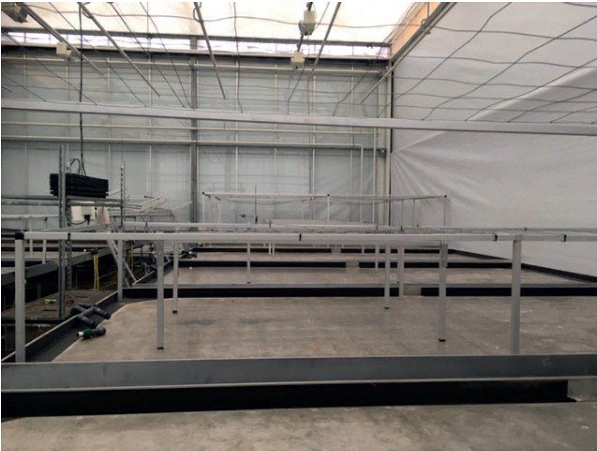
Figure 2 Aluminium frames built to support the heavy Electrochromic Glass panes and the reference glass panes.
