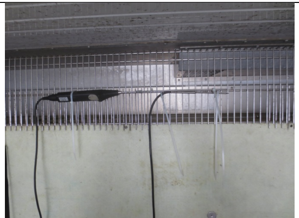
Fig. 2, one USDA probe and reference temperature sensors mounted in return air grid.
