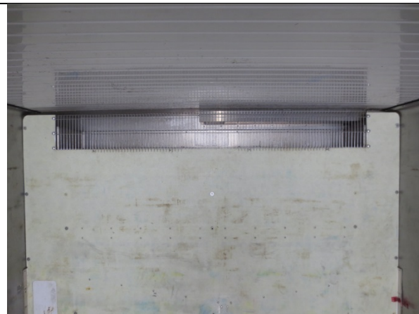
Fig. 1, return air grid
