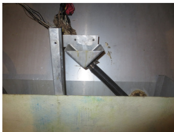
Fig. 3, original (single) drain pan, directly connected to drain line.
