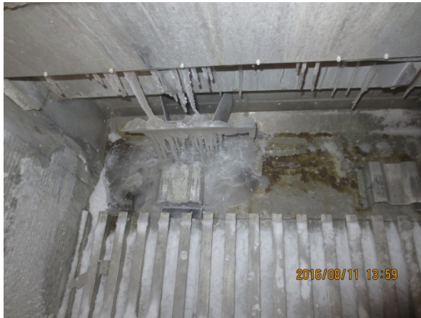
Fig. 25, ice on left-side of floor at end of test 1.
