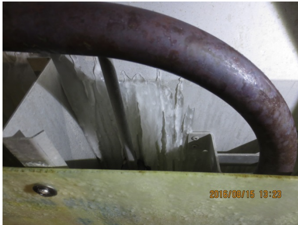
Fig. 29, icicles attached to the unit's front panel at end of test 2.
