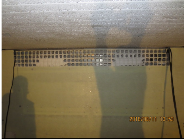
Fig. 21, return air grid at end of test 1, just before defrost start.
