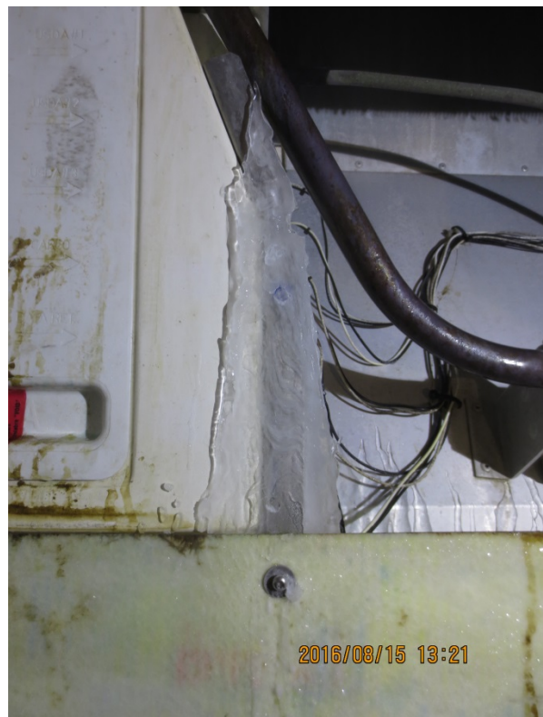
Fig. 28, ice behind unit's upper rear panel at far-left side at end of test 2.
