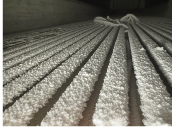
Fig. 22, snow covered floor at end of test 1.
