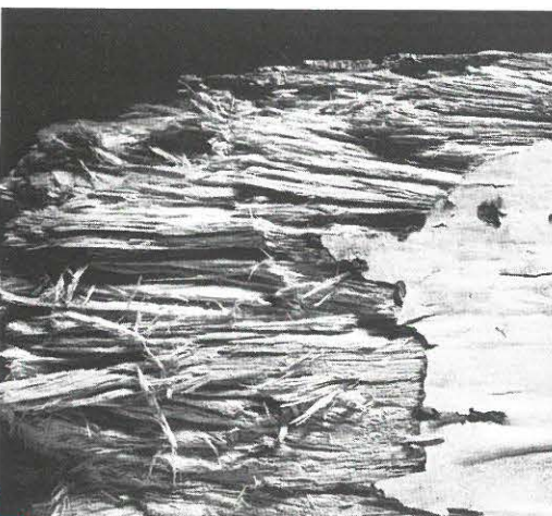
Typical white rot damage to timber
