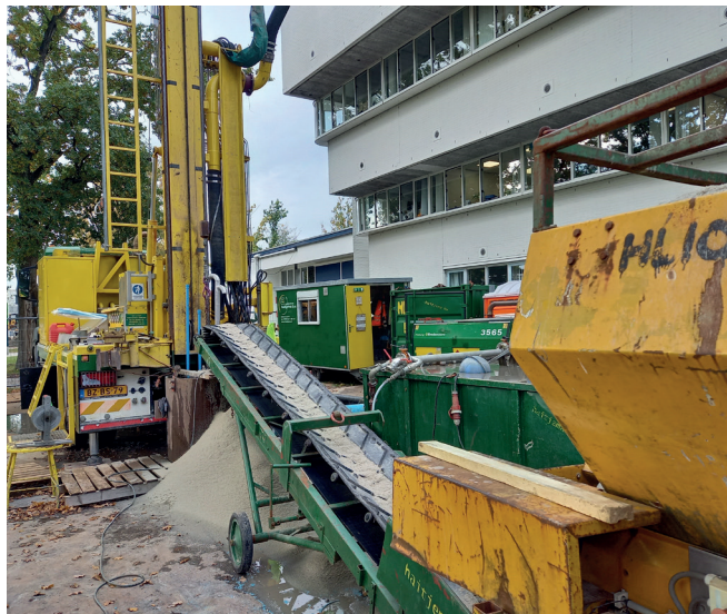
Fig. 7: The shaft is backfilled with sand or micolite depending on the layer.
