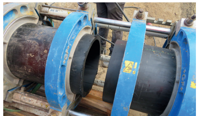
Fig. 4: The pipe ends are planed off parallel and can now be welded together.
