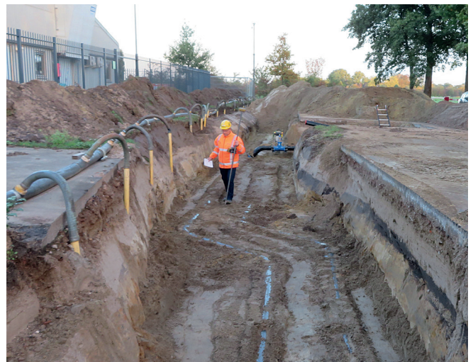
Fig. 7: Once everything is in position, Thijs surveys the exact location of the pipes, every weld and all the valves, couplers and T-pieces.
