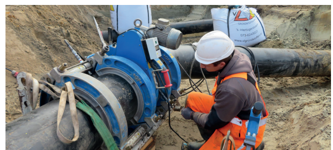
Fig. 5: The hot mirror is placed between the pipes, after which these can be welded to each other.
