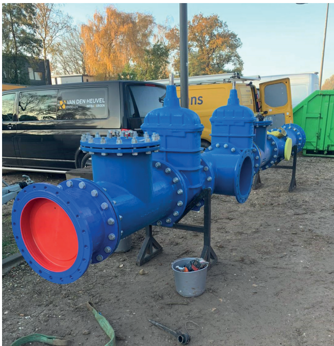
Fig. 1: The assemblies are put together in the depot. This assembly weighs approximately 2200 kilos.
