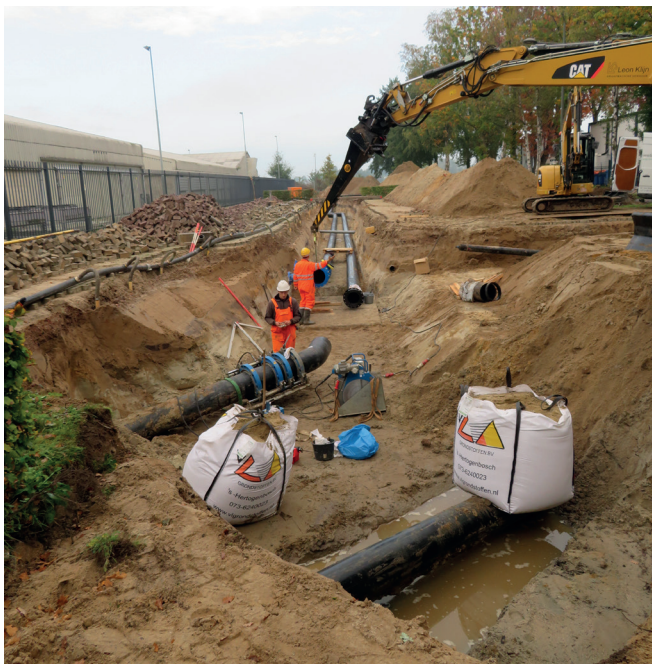
Fig. 2: Bigbags are used to bend the pipes installed by HDD to the correct depth.
