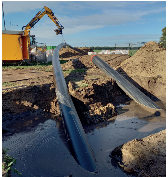
Fig. 6: During pulling in, the pipe is guided by a crane to reduce friction.
