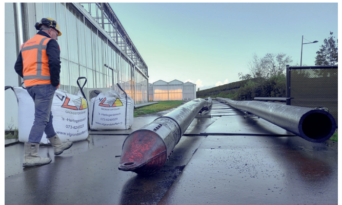
Fig. 5: Alongside Radix Serre's greenhouses, two 450 mm pipes 300 m long are lying on rollers ready to be pulled in; the left pipe has already been fitted with a puller head.
