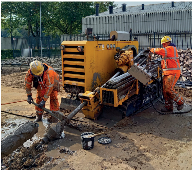
Fig. 4: The pulled-in pipe has resurfaced at the entry, so the puller head can be removed and the reamer can be unscrewed.
