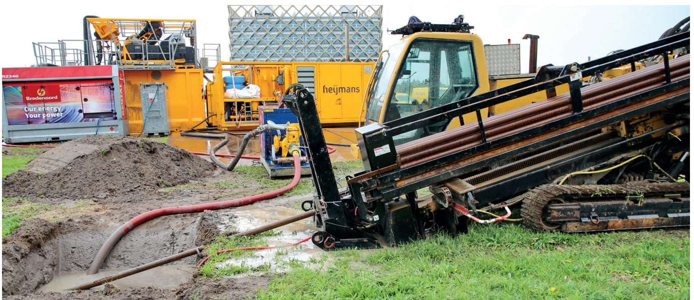
Fig. 1: A drilling rigs at the entry pit. This heavy machine automatically connects the extension rods; with lighter machines, this happens manually
