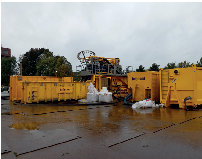
Fig. 2: In one container, the bentonite is prepared and pumped into the shaft. The machine separates the bentonite-sand mixture coming out using vibrating screens and distributes it among the other containers.
