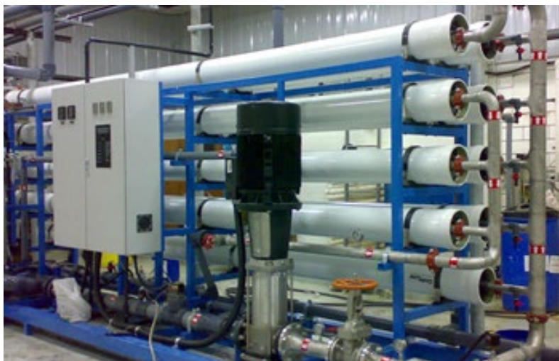
Figure 2.4 RO-unit with 9 tubes holding 4 membrane elements each (Photo: WLR).
