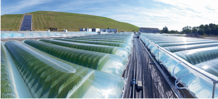
Fig. 4-1 Proviron plant in Antwerp 2015, comprising 120 reactors with 4 control units, each operating 30 reactors in parallel. A feed container in turn services multiple units. The first unit with 20 reactors was operating through 2012
