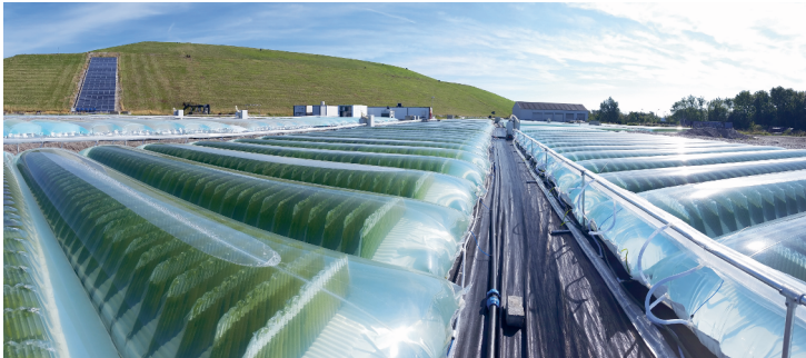
Fig. 1-5 The Proviron flat plate photobioreactor plant, installed on the municipal solid waste treatment plant, Hooghe Maey in Antwerp in 2015. The hills in the back of the picture are membrane covered, solid organic waste heaps, covered with a membrane. They produce biogas that is combusted in gas motor driven, electrical power generators. Photograph: courtesy of Proviron.
