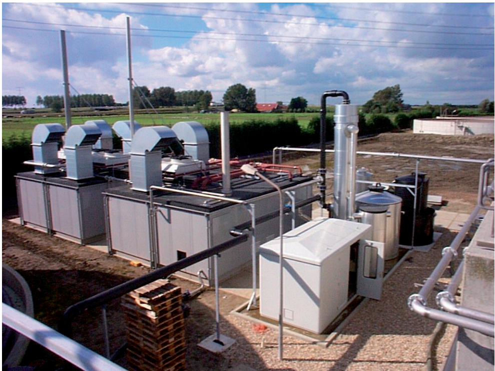
Figure 7: THIOPAQ installation in the Netherlands (courtesy of Paques).
