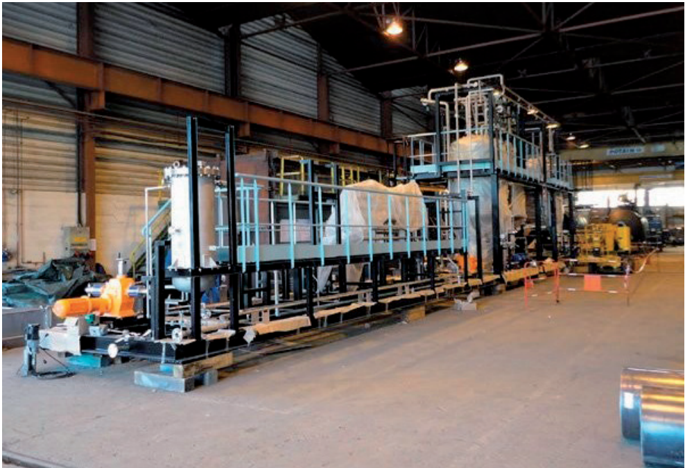
Figure 4: Supercritical water oxidation plant in France.
