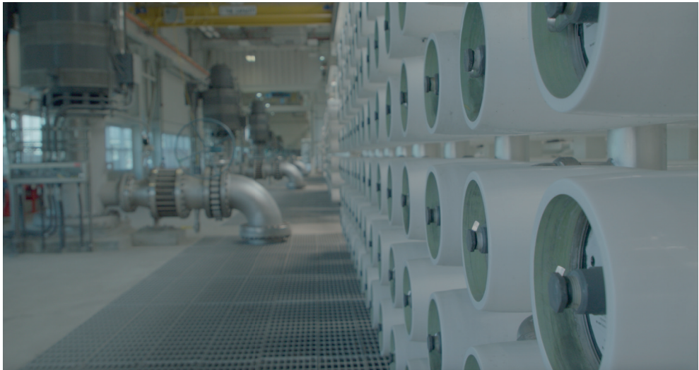
Figure 6: Reverse Osmosis membrane modules at Orange County, California (courtesy of Brave Blue World foundation).
