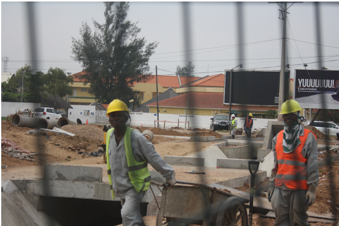
Construction workers building a new drainage system connecting the upper heights of the city (Polana Caniço) with the Marginal. They began to recognise me, as I passed by them almost every day on my walk up and down my sites, and would ask for their picture to be taken.
