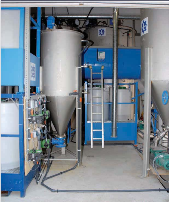
Figure 7 - Anaerobic treatment of black waste(water) in The Netherlands , 32 houses (Meulman, Landustrie BV).
