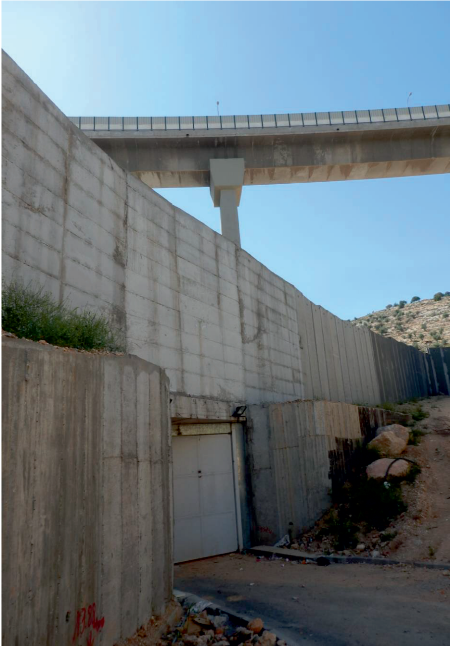
Figure P.4: The Wall in Bir Ouna, with The Tunnels highway passing over it (source: Rijke, May 2017).
