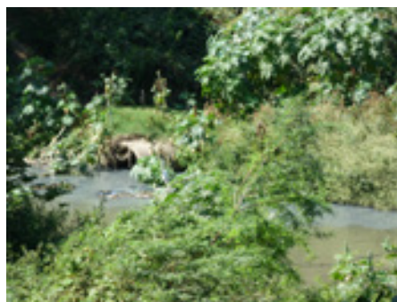
Untreated piped outfall
