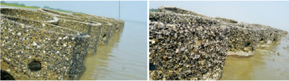
Fig. 1.4 Eco-engineered concrete units with recruited oysters. Note the oyster growth on deployed oyster reef units after just eight months (left), and 2 years (right) post-deployment at the offshore island of Kutubdia.
