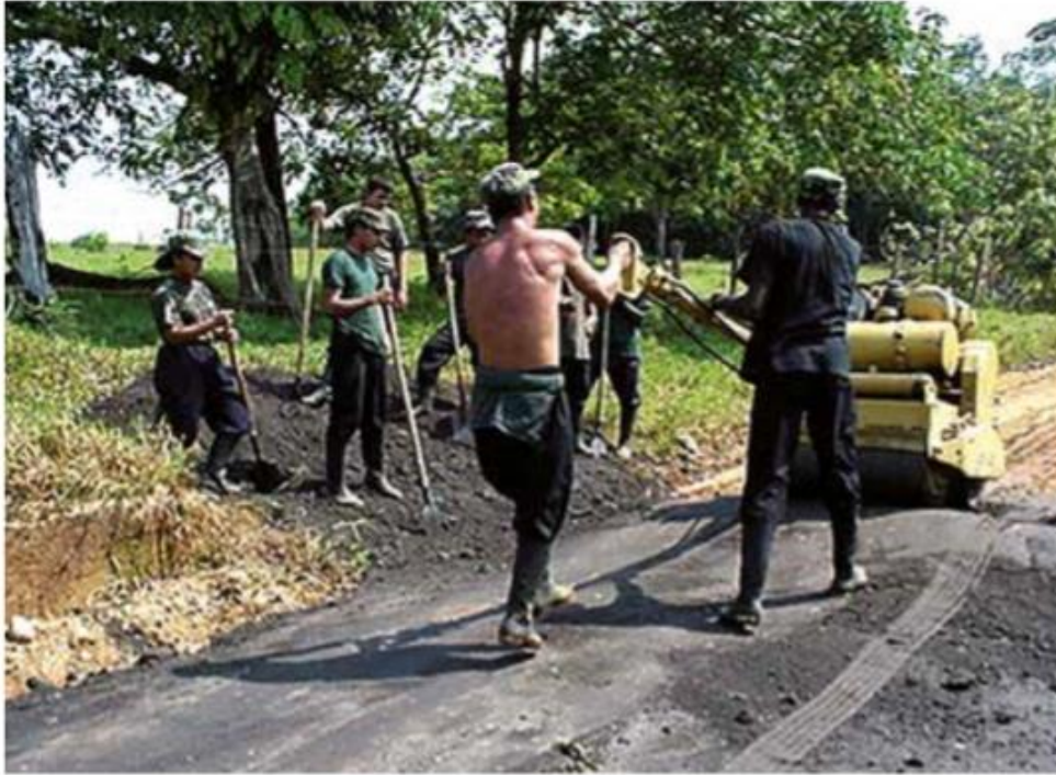
Figure 4.7 Fighters working on the construction of a road in the Caguan region. (Viva, Candelaria y Gonzalo, N., 2014). Re-printed with permission of the authors.
