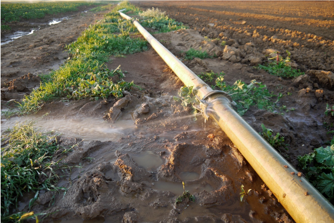
Fig. 10. An example of leakage of the supply pipe of a sprinkler system in the Mediterranean region.
