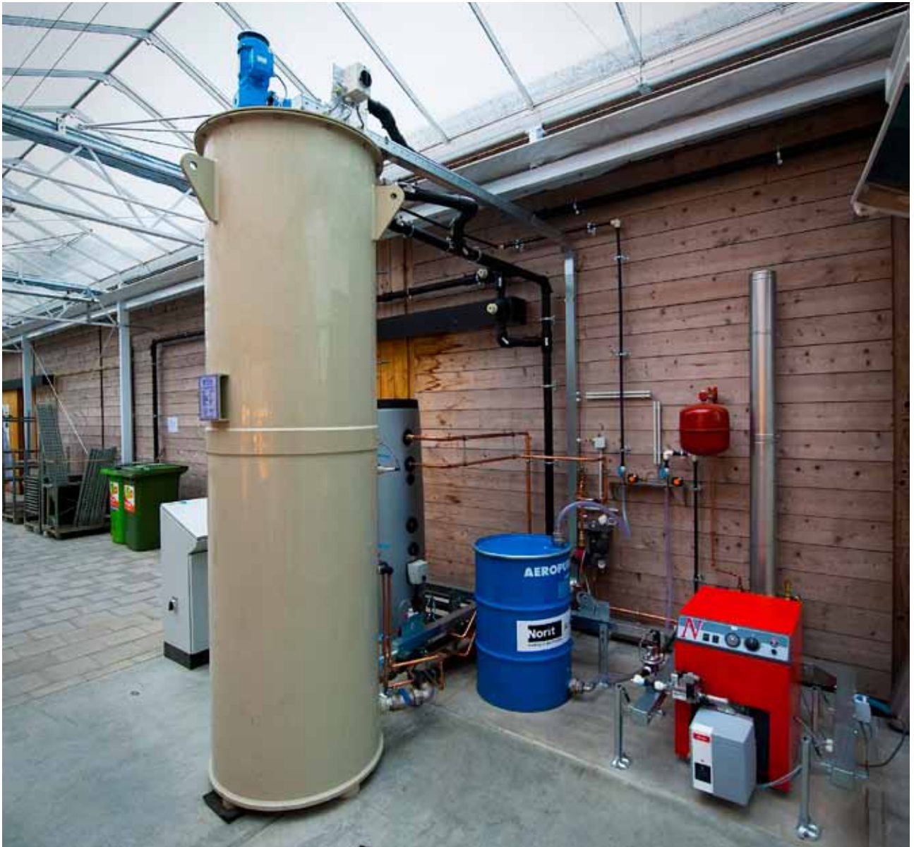
Anaerobic digester for purifying 'black water' and producing biogas, at the NIOO in Wageningen.
