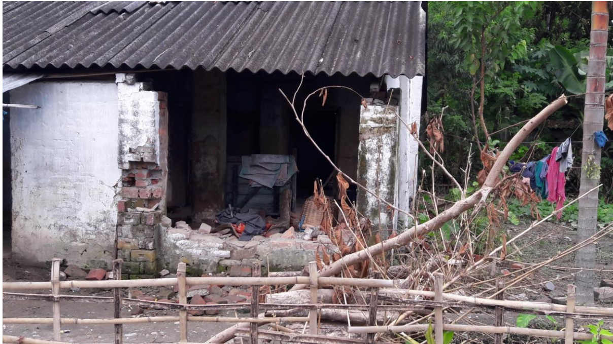
Figure 3 Dilapidated housing, Hattigor 2017. Source: Accountabilitea project
