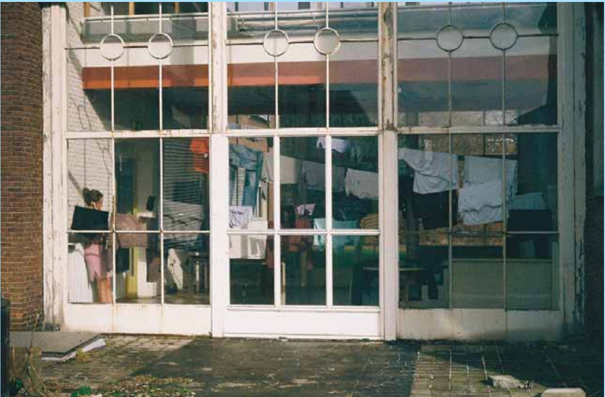
Although the old IPO building is not fit for human habitation, the students living there manage to have a good time. / photo MW
