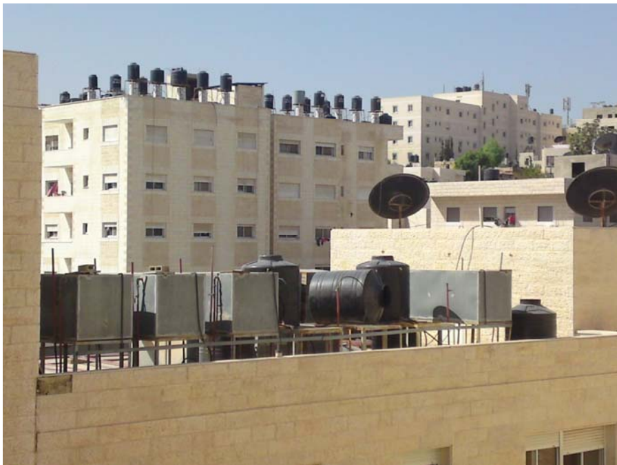
Figure 7. Rooftop water tanks in the village of Abu Dis. Own photo, taken October 2015.
