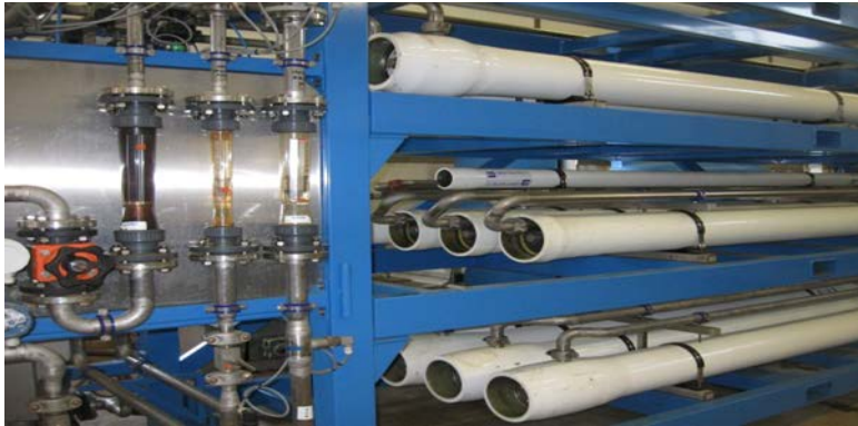
Figure 12 Reverse osmosis installation for production of NK-concentrate.
