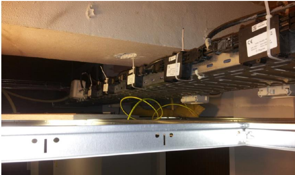
Figure 11: Electricity meter installation at Student hotel
