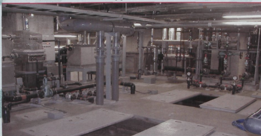
Overview Kubota installation in the Ebisu building (photo DHV Water).
