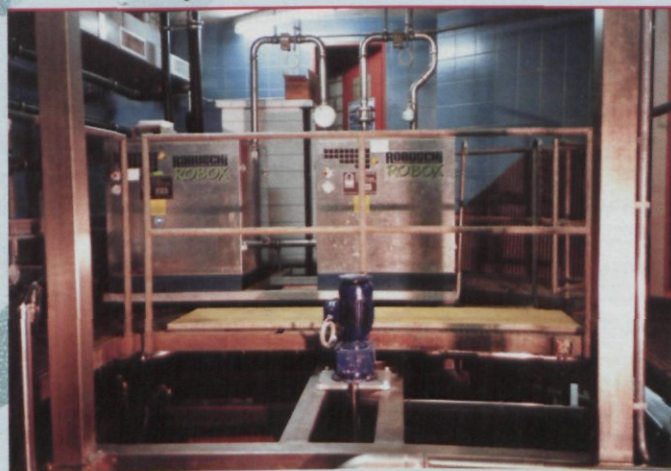
Wastewater treatment plant at Säntis.
