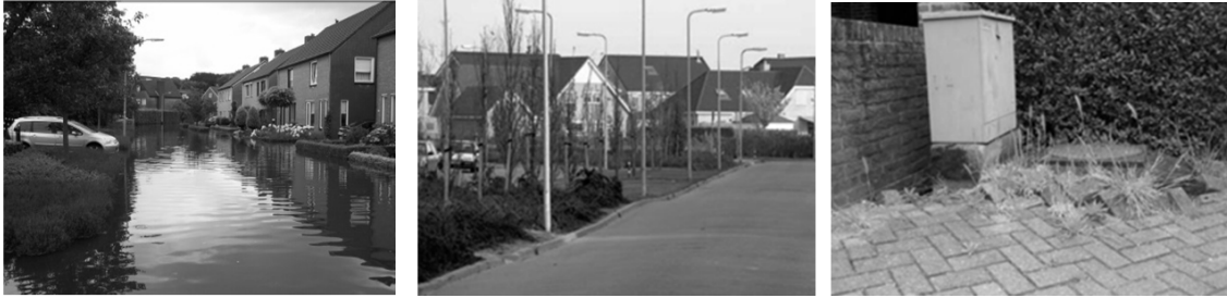
Figure 7 Problems associated with building on peatland, examples from the Netherlands: flooding (left); subsidence of roads (middle), and; subsidence of sewerage mains (right) (Photos: Deltares, 2008).
