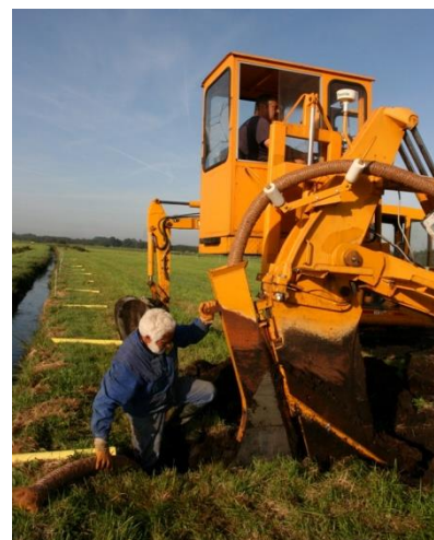
Fig. 1: Installation of subsurface drains for subirrigation in grassland on peat soil (Photo: B. Tiemeyer)
