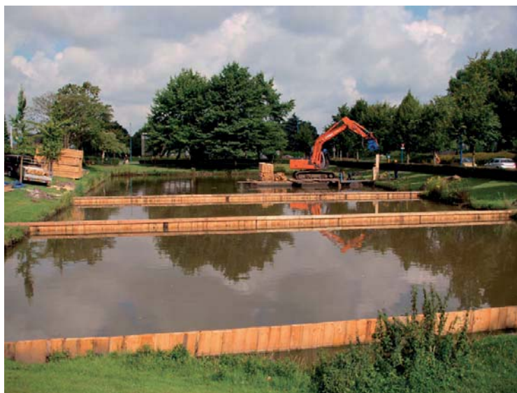
Fig. 3.C.1: Construction of compartments separated by wooden sheet pilings in pond Dongen (28 July 2009).
