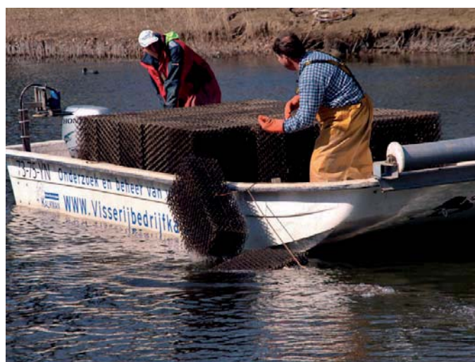
Fig. 1.4: Construction of a reef, using crates overgrown with juvenile herbivorous mussels ( Dreissena rostriformis bugensis ) in an urban pond in the city of Breda (The Netherlands, 2 April 2013).
