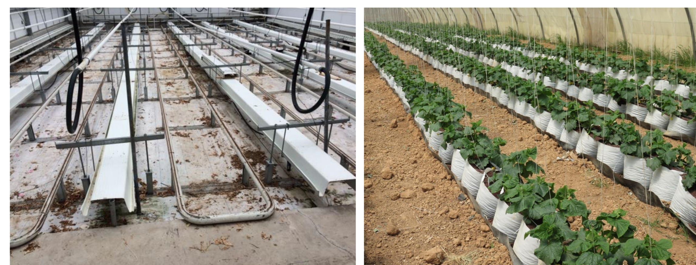
Figure 3: Troughs for a 2-row system (left), in combination with a transport/heating system in the path.
