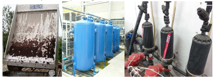
Figure 2: Filters for coarse materials, such as potting composts (left), sand filter (middle) and disk filter (right) to be used before disinfection.
