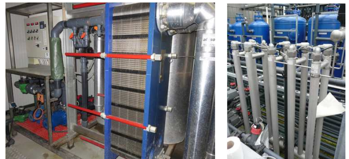
Figure 6: Left Heat Treatment installation, right Low Pressure UV light installation.
