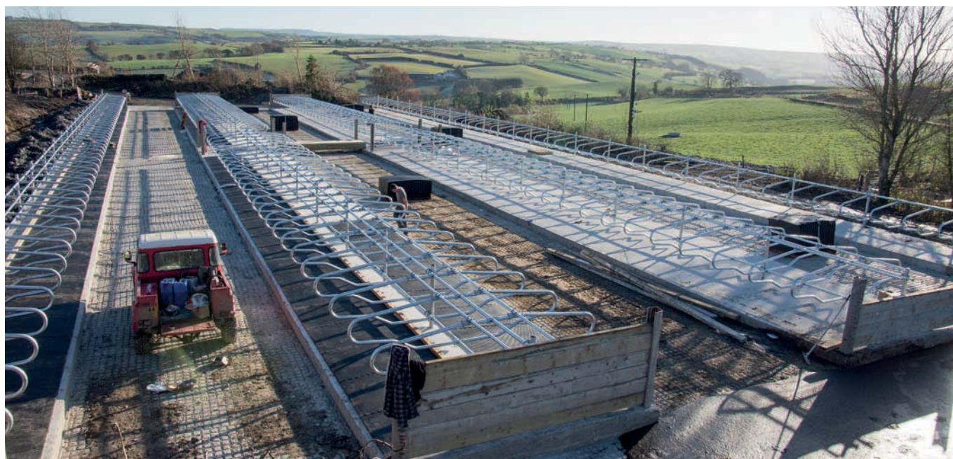
Left: North Wales-based unit offers wonderful views and a fantastic share-farming opportunity Below: cubicle housing for the expanding herd is under construction
