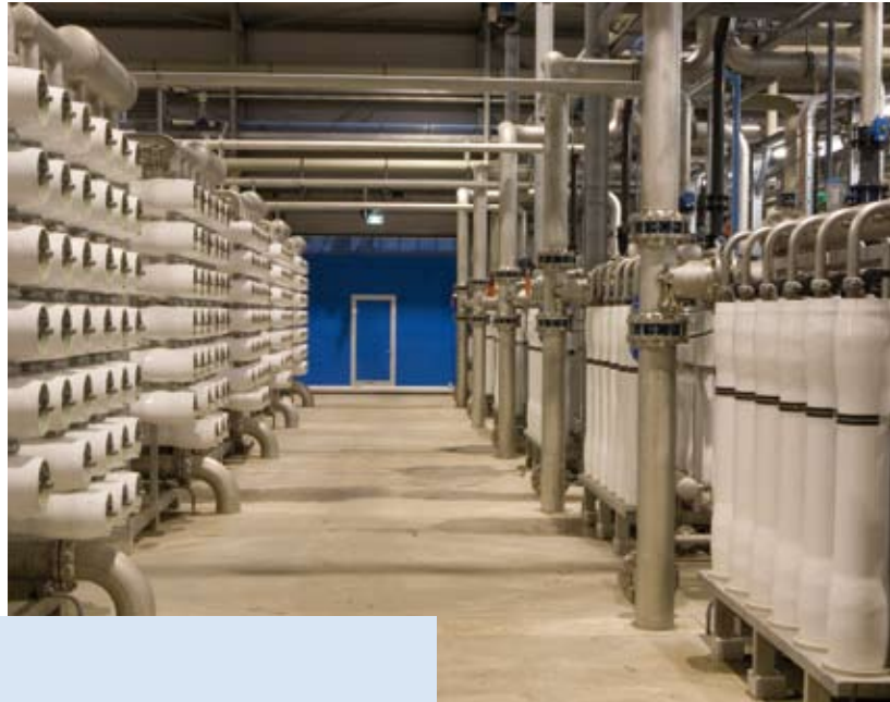
Demiwaterinstallatie DWP in Botlek (foto: Logisticon)
