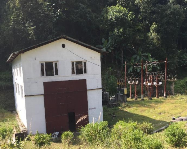
Figure 5 Power house of Middle PHEME HPP (picture made by author during field work in November 2015)
