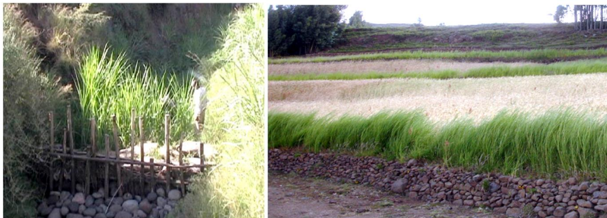
Figure 3.7 Examples of the combined application of vegetative and structural measures for sediment trapping northwest Ethiopia (photo by Mulatie Mekonnen): check dams combined with grass (left) and terrace combined with grass strip on top (right)
