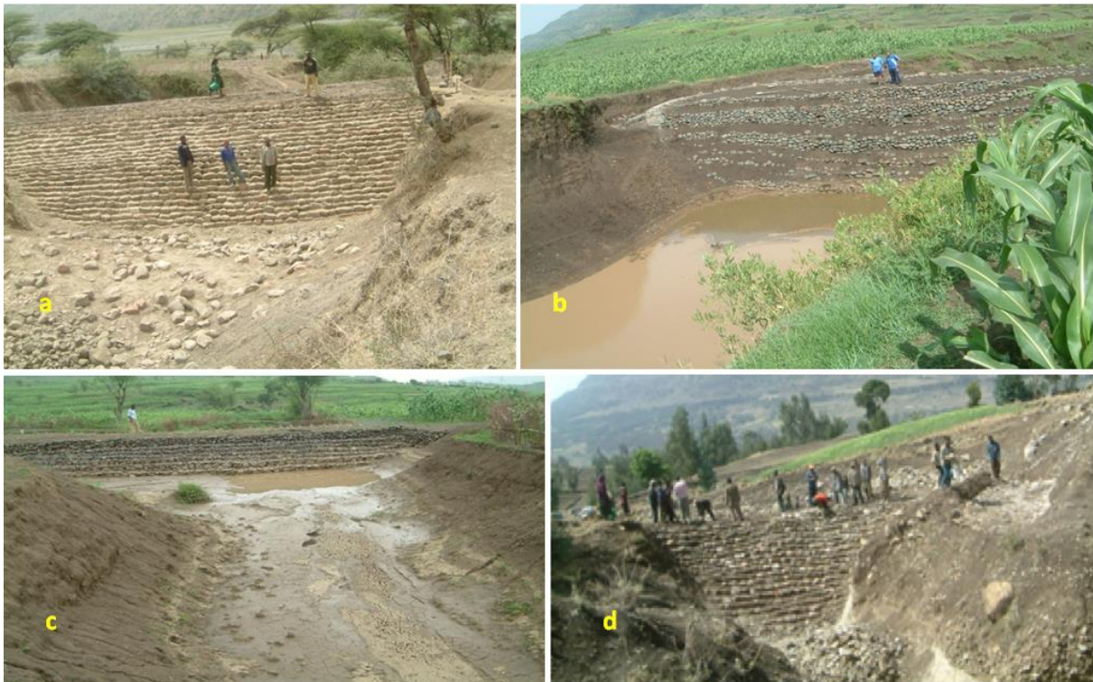
Figure 5.2 Examples of SSDs constructed in the Amhara region, Ethiopia (a) Delanta, (b) Kobo, (c) Bati and (d) Kutaber (Photos by Mulatie Mekonnen)
