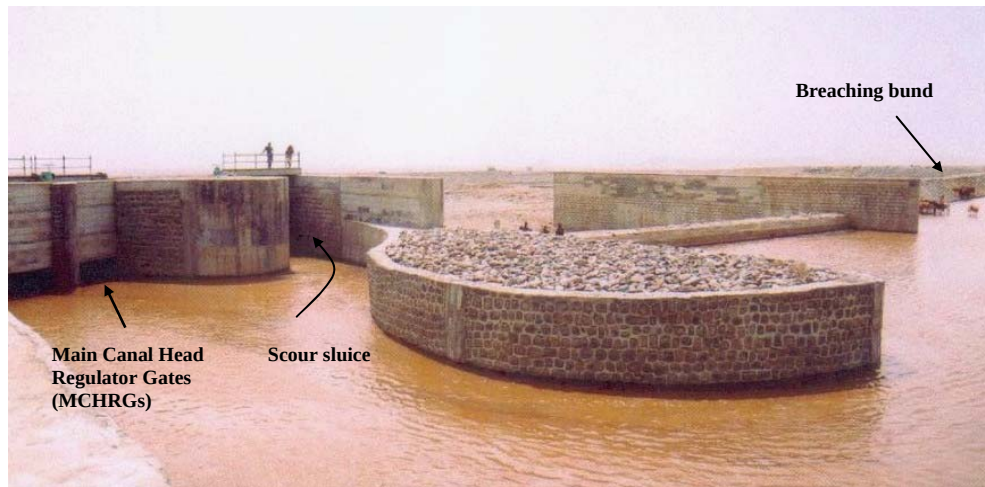
Figure 4.10 The Wadi Laba modern headwork
