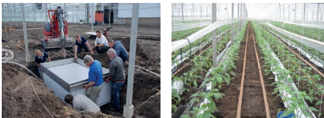
Figure 23 Installation of a lysimeter in a greenhouse (A) and after installation with a young sweet pepper crop (B) (photos: Wim Voogt).
