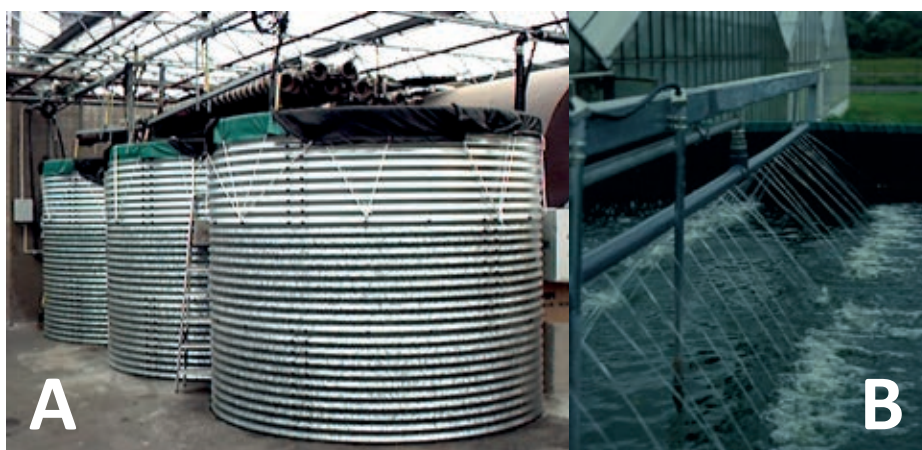
Figure 16 Examples for decontamination of irrigation water by filtering. A: Slow filter consisting of three units, (i) collection tank for drainage water, (ii) slow filter unit and (iii) tank for treated water (Österlen tomat, Glimmingehus, Sweden); B: sprinkler unit to the slow filter (Kienzler, Gensingen, Germany). (photos A: Beatrix Alsanius; B: Walter Wohanka) 2 .
